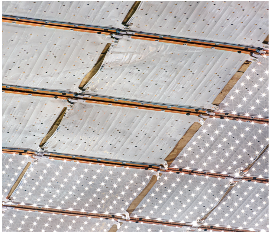
TILE Interior mounted directly to the plywood ceiling without heat sinks
